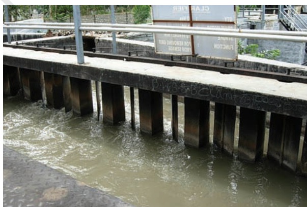
Fig. 18.4 Grit and sand removal tank
